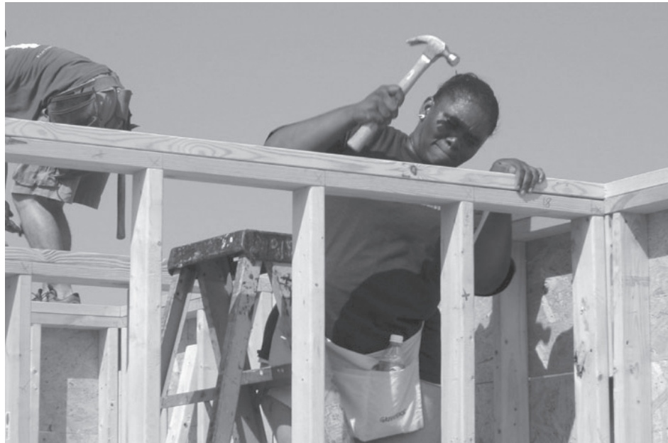
Building a PVC-free house in the 9th Ward of New Orleans, sponsored by Greenpeace, the New Orleans Area Habitat for Humanity and the Healthy Building Network.
